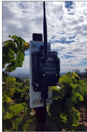
To transmit its measurements, each moisture sensor is wired to a Banner Engineering SureCross 900 MHz radio.
